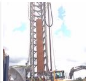
Class I Injection Well capable of receiving 20MGD of non-toxic wastewater
